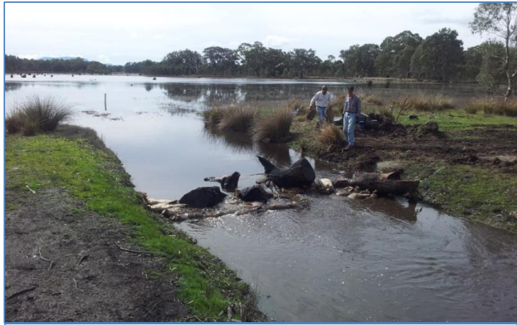
The First Step – Constructing a hessian sandbag and log bund to reduce flow rate and (to a lesser extent) depth in the channel.
