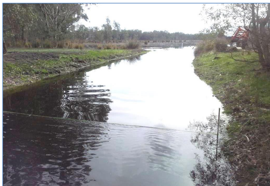
Site conditions upon arrival at the site on the 26th August looking towards Gooseneck Swamp from the drain. The pegs indicate the proposed location of the sandbag weir, and the string-line was used to monitor the downstream change in channel water level in response to the works throughout the day,
