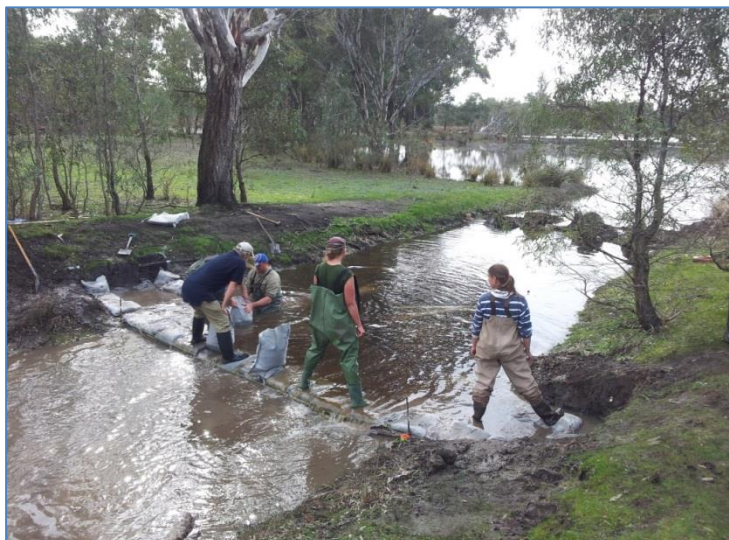
The sandbag crew succeeding in getting the weir to reach the height of the channel water level. Notice the minor drop in water level downstream as the weir under construction starts to hold back water.
