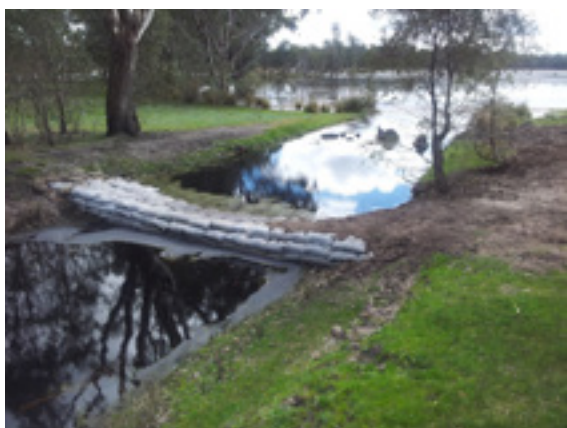
The Gooseneck Swamp Restoration Trial Structure was installed in August 2013 and is situated in the artificial outlet drain from the swamp (© Copyright, Mark Bachmann)
