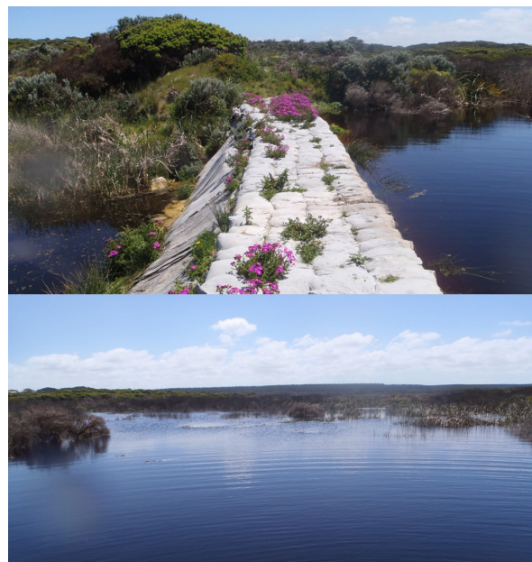
Figure 1—from top: The trial structure at Nobles Rocks built of over 7000 sand bags and recreated aquatic habitat upstream of the weir. (Lauren Veale)
