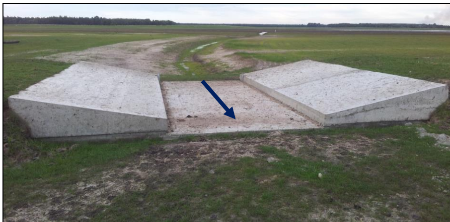
Example NGT structure near Dunkeld, which sets a new restored “fixed” sill level (maximum retention height) for this substantial wetland (background), but maintains the existing artificial drain alignment.
