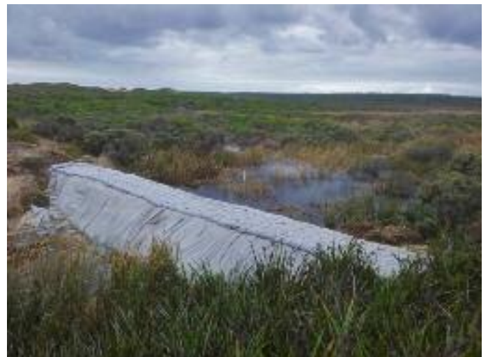
The phase 3 trial structure (foreground) has begun to regulate wetland levels in Long Swamp (background) by restricting flows from the Nobles Rocks outlet. Photo: Mark Bachmann
