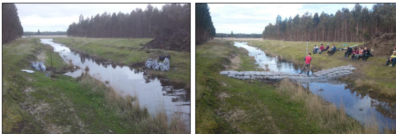
Before (left) and after (right) the construction of the trial structure in 2014 - looking upstream towards Walker Swamp
