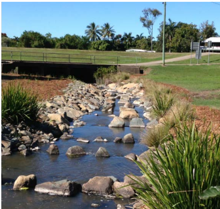
Figure 51. Example of a rock ramp fishway in Mackay, Queensland (photo: Catchment Solutions (2022)).
