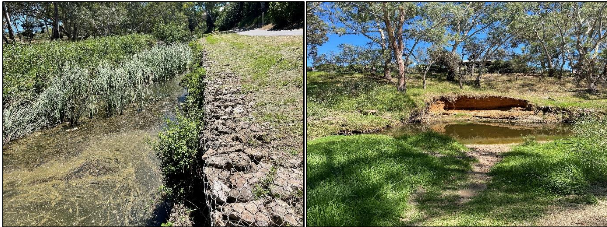
Figure 12. Bank condition in section 4.
